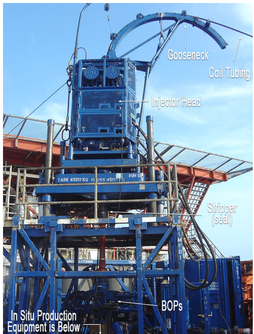
Figure 32- Coiled Tubing Injector Head on a Platform
